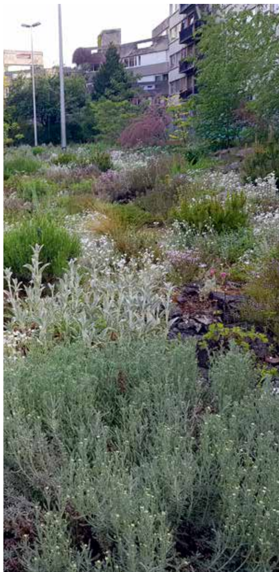
Concrete crushing and planting on a former parking lot in the city of Aubervilliers, France ©Wagon landscaping
